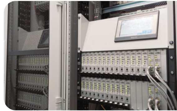
ESSO-M-2 tower equipment
