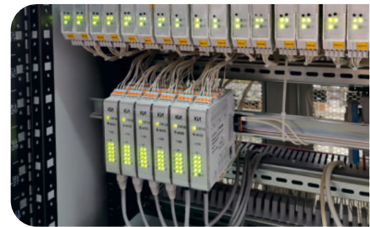
ESSO-ILS tower equipment
