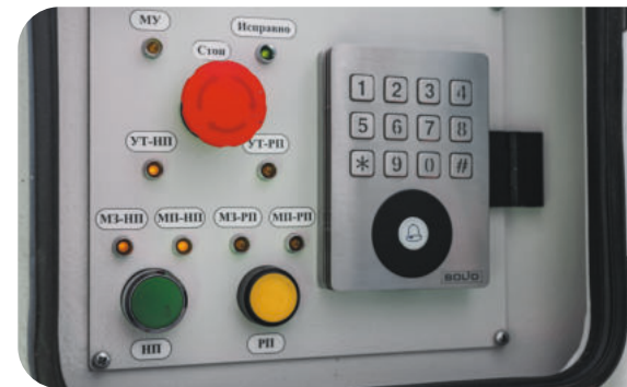
Local Control Panel
