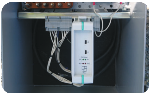
BOS Signal Processing Unit
