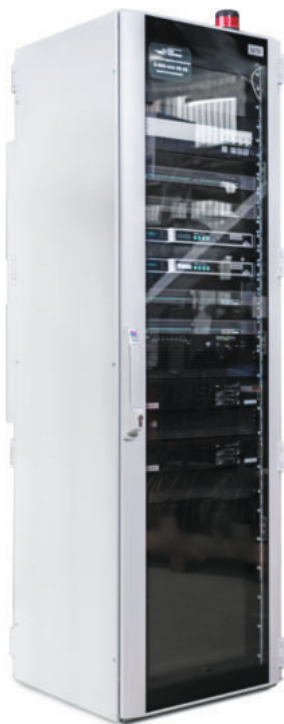
ShTK Communications Cabinet
